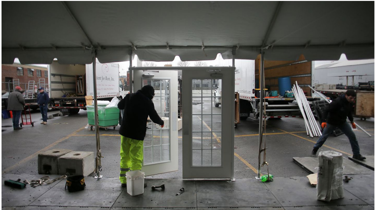
Crews erected tents last month to serve homeless people during the COVID-19 crisis behind a Southhampton Street shelter. The heated tents will have bathrooms and showers, and space for 40 beds so infected homeless people can be separated from the shelter community and get the care they need. LANE TURNER/GLOBE STAFF
